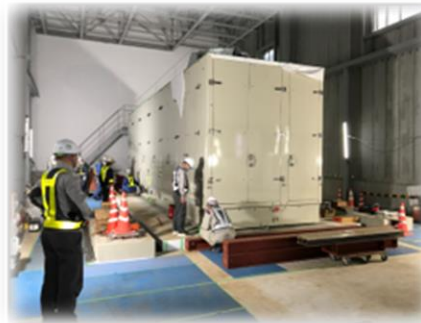
Cogeneration Plant at Misawa AB
